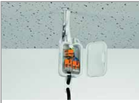
Pendant light connection in suspended ceilings
